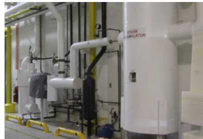
The Oxford, Pennsylvania bakery reuses heat generated by ovens to heat water and other areas of the facility.
